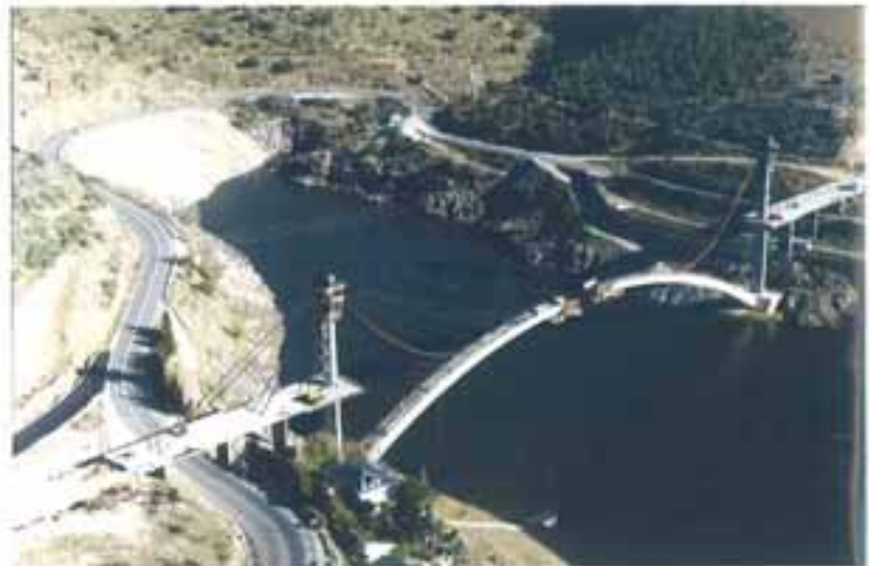
Foto 3. Vistas del arco durante procedimiento constructivo. Picture 3 Views of the arch during the construction procedure.
