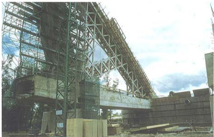
Foto 4. Vista de la cimbra de la vela inclinada. Figure 4. View of the centering used for the construction of the inclined sail.
