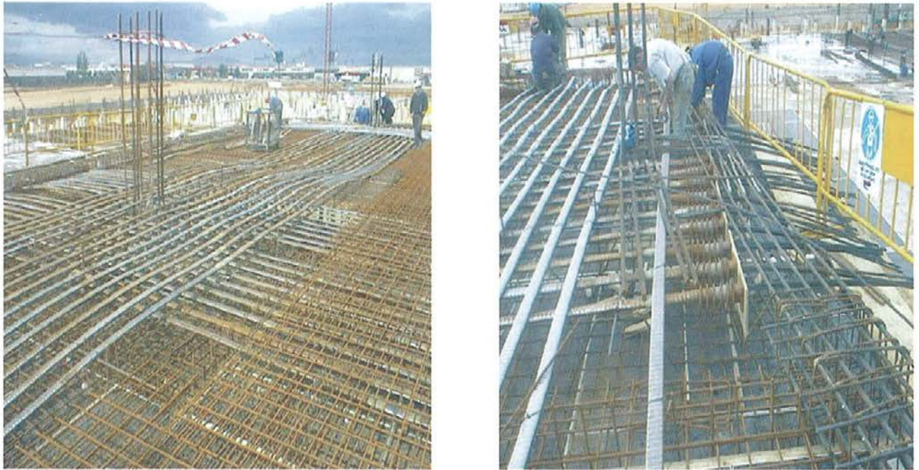
Figura 17. Vista general pretensado de planta primera. Figure 17. General view of prestressed slab.
