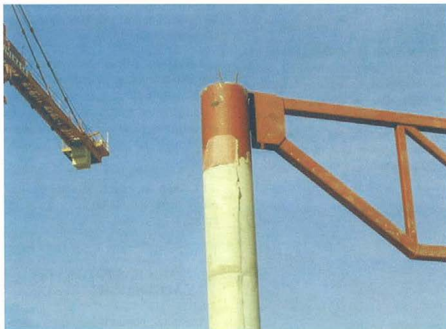
Figura 4. Detalle cabeza pilar con collarín. Figure 4. Detail of union between column and roof structure.
