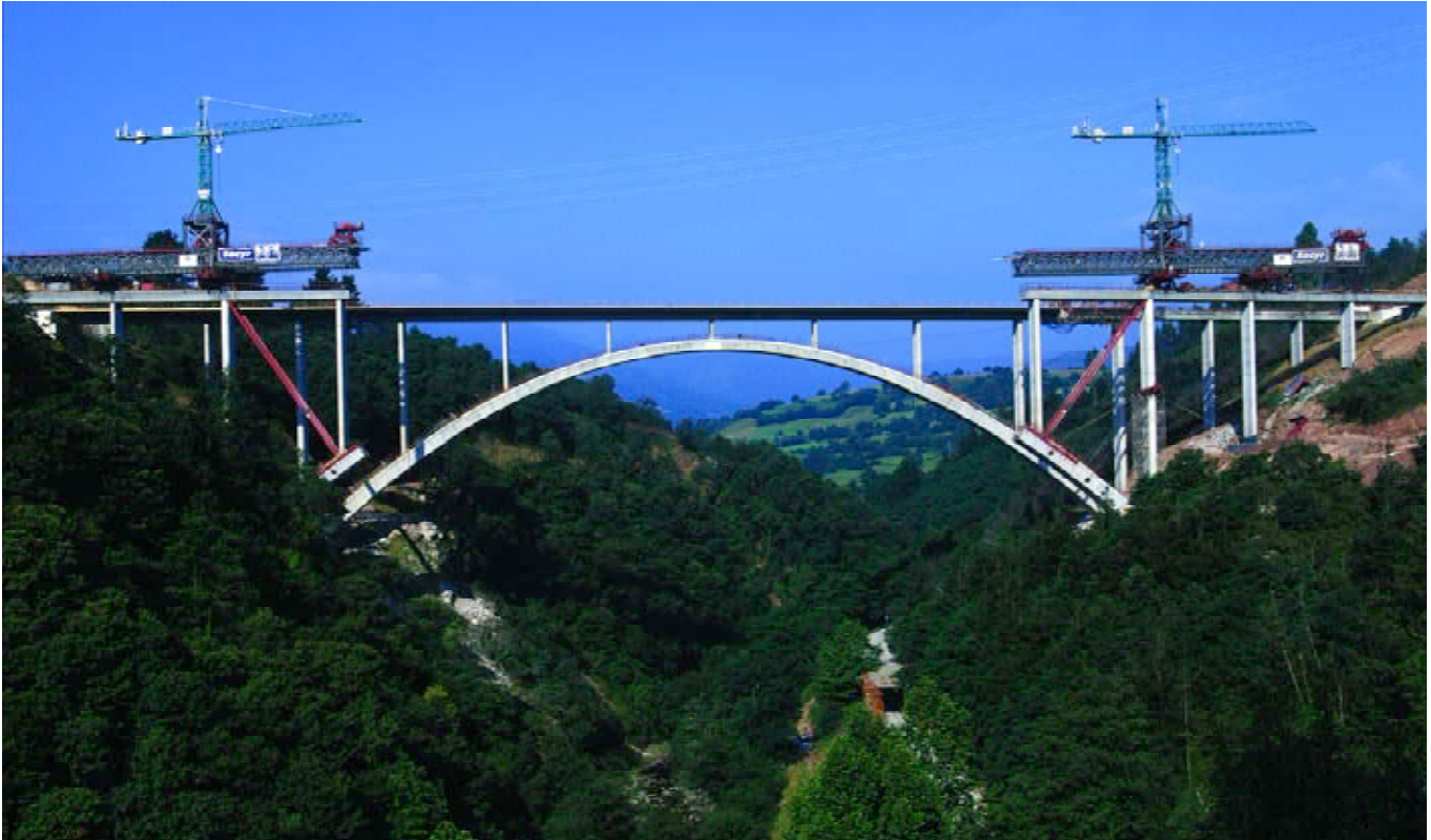
Figura 16. Alzado general del puente durante la construcción. Figure 16. General elevation of the bridge during construction.
