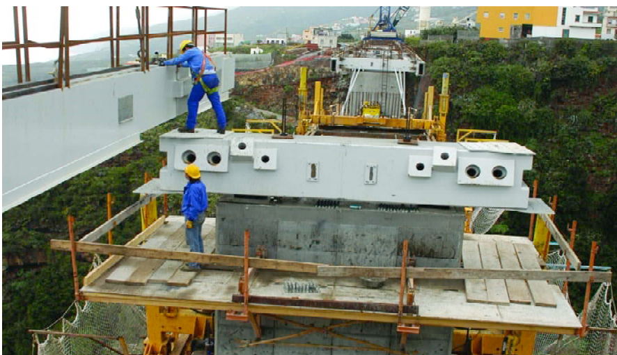
Figura 15. Rostro de pila. Figure 15. Column bracing.
