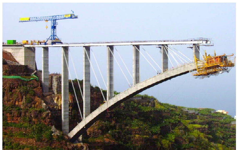
Figura 10. Avance en voladizo con diagonales temporales. Figure 10. Progress in cantilever with temporary diagonals.
