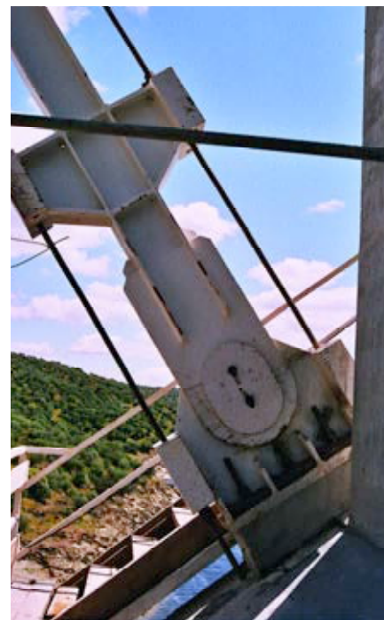
Fig.42. Detalle de tesado de diagonal rígida. Fig.42. Detail of rigid diagonal tensioning.
