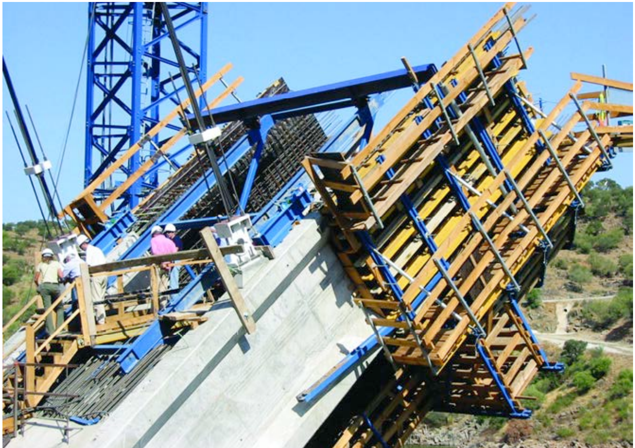
Fig.33. Carro de avance en voladizo para el arco, con tirantes auxiliares. Fig.33. Cantilever advancing carriage for the arch, with auxiliary stays.
