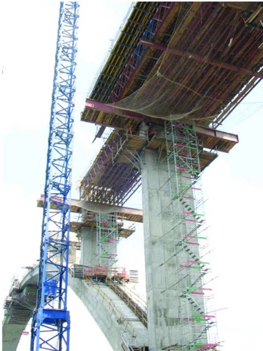
Fig.18. Ejecución del tablero mediante autocimbra. Fig.18. Building the deck with scaffolding truss.
