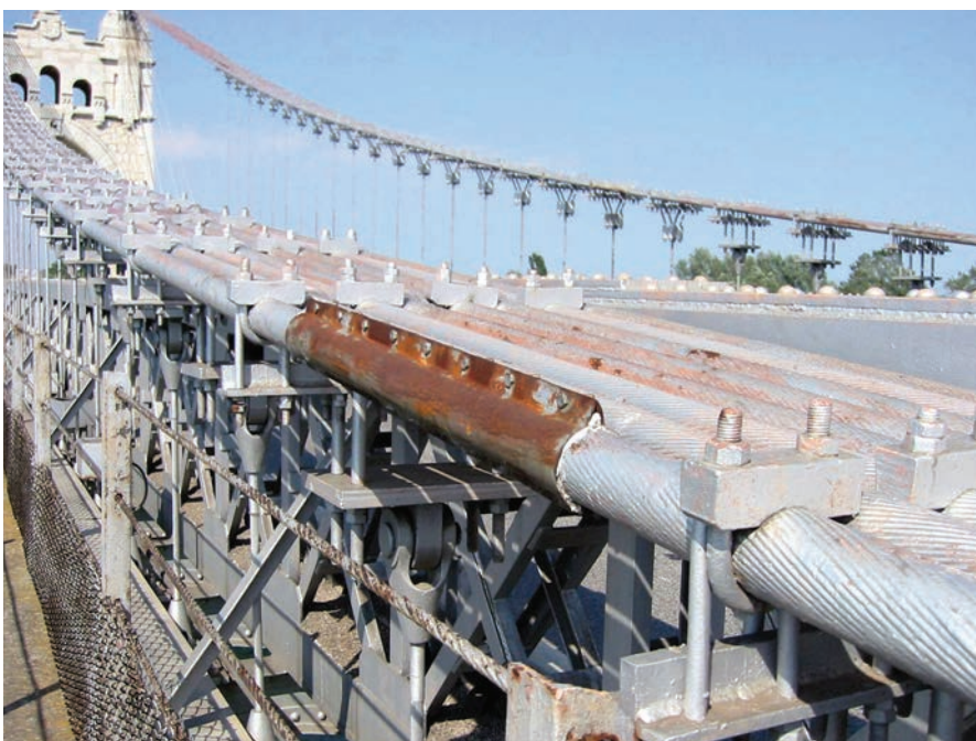
Figura 17. Cables reparados en 1972. Figure 17. Cables repaired in 1972.
