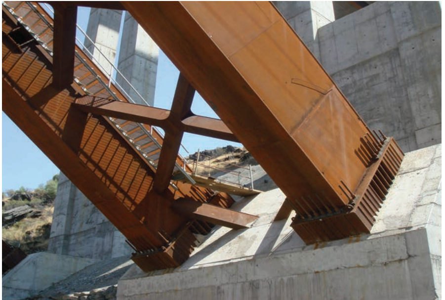
Figura 36. Empotramiento del arco en su base. Figure 36. Fixing the arch in its base.
