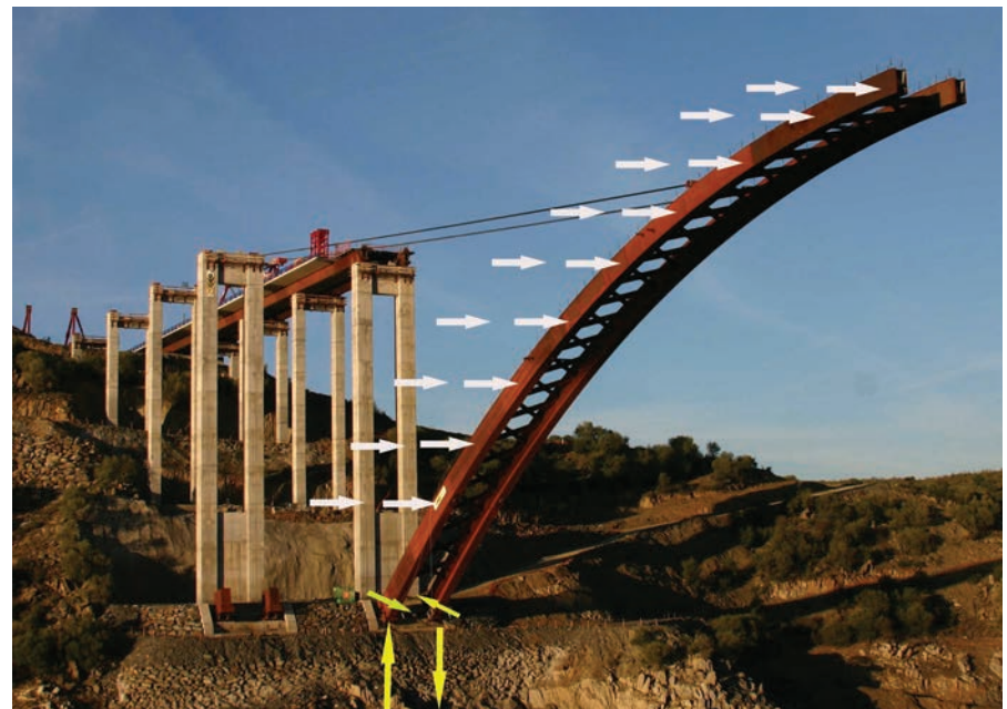
Figura 50. Efecto del viento lateral sobre un semiarco durante la maniobra de abatimiento. Figure 50. Side wind effect on one semi-arch during the swivel lowering operation.
