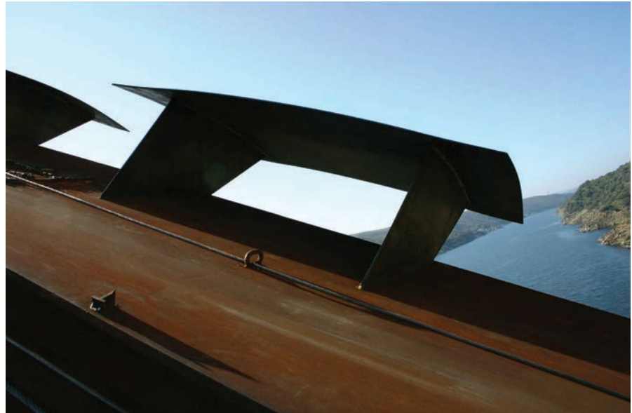
Figura 58. Deflector. Detalle. Figure 58. Guide vane. Detail.
