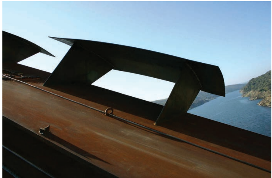
Figura 58. Deflector. Detalle. Figure 58. Guide vane. Detail.
