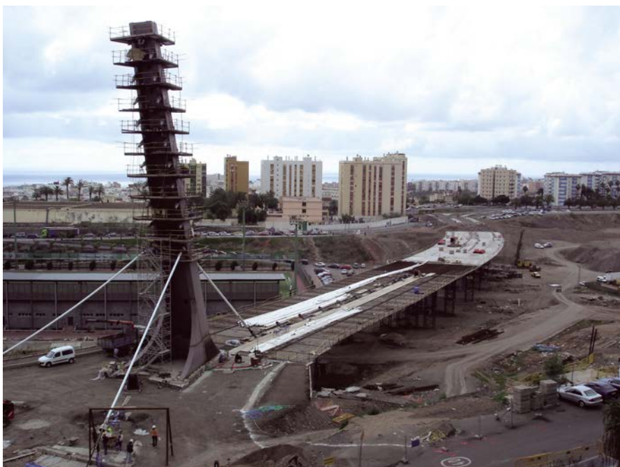
Figura 35. Montaje de la primera terna de tirantes. Figure 35. Assembly of the first batch of stays.
