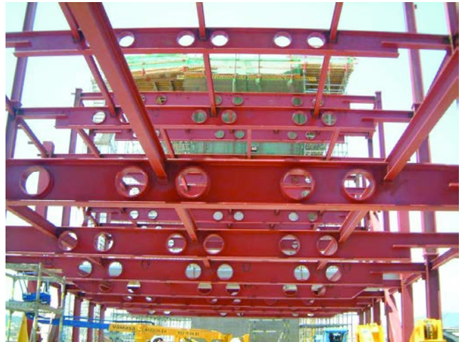
Figura 28. Estructura de vigas de una planta del Portaaviones. Figure 28. Beam structure on one floor of the Aircraft-carrier building.
