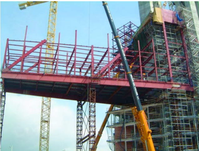
Figura 18. Ejecución del portaaviones en fase 3. Figure 18. Stage 3 construction of the Aircraft-carrier building.
