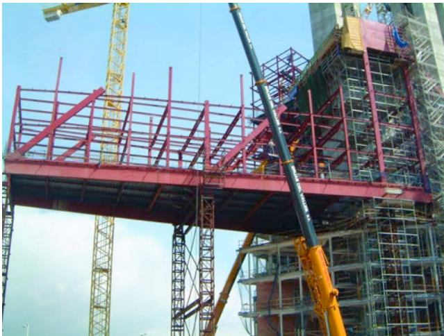
Figura 18. Ejecución del portaaviones en fase 3. Figure 18. Stage 3 construction of the Aircraft-carrier building.
