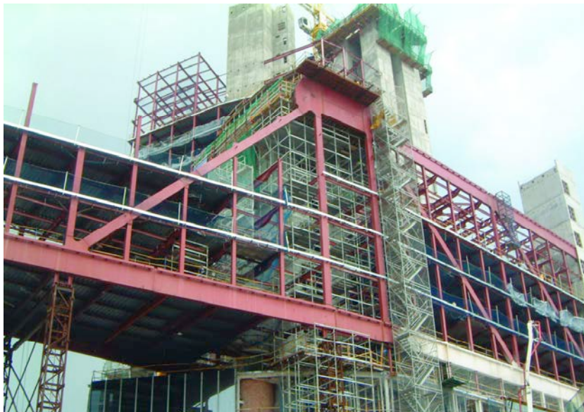
Figura 22. Vista de la ejecución de la fase 4 del Portaaviones. Figure 22. View of stage 4 construction of the Aircraft-carrier building.
