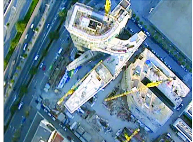
Figura 32. Vista aérea en planta durante la construcción. Figure 32. Aerial view of the site during construction.
