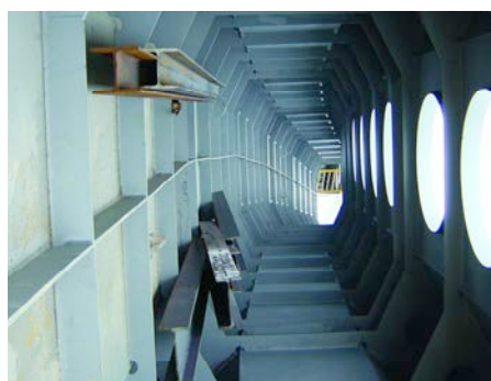
Figura 43. Aspecto del pasillo interior reforzado con los rigidizadores. Figure 43. Appearance of the interior corridor with the reinforcement of the stiffeners.
