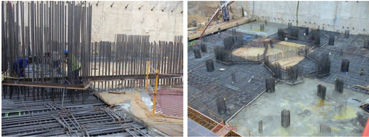
Figura 9. Plantilla de colocación de armado de núcleo y vista general del hormigonado de la segunda tongada de losa. Figure 9. Mould for the installation of the core reinforcement and general view of the concreting of the second concrete lift of the slab.
