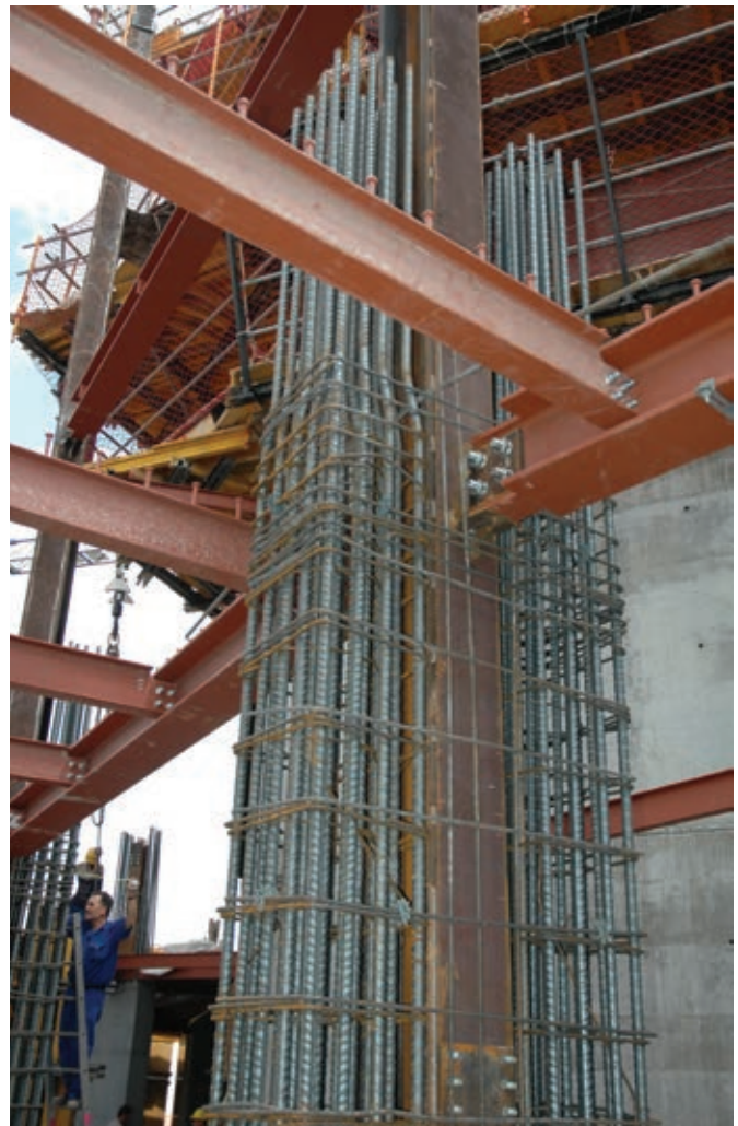
Figura 9. Soporte mixto densamente armado en la zona baja de la torre preparado para la colocación del encofrado. Figure 9. Joints between sections of steel supports, capable of withstanding the wind loads during construction.
