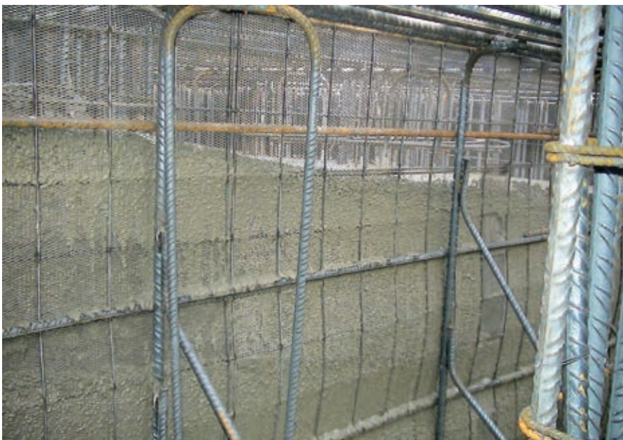
Figura 5. Detalle de junta vertical con nervomental. Figure 5. Detail of vertical joint with nervomental (metallic reinforcement).
