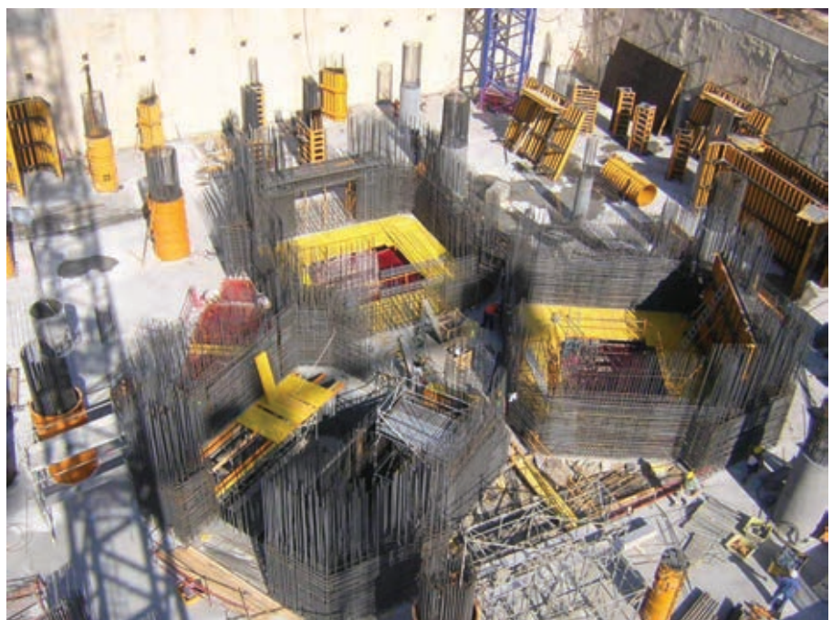
Figura 13. Vista general de armado y encofrado de núcleo y soportes. Figure 13 General view of the reinforcement and formwork of the core and supports
