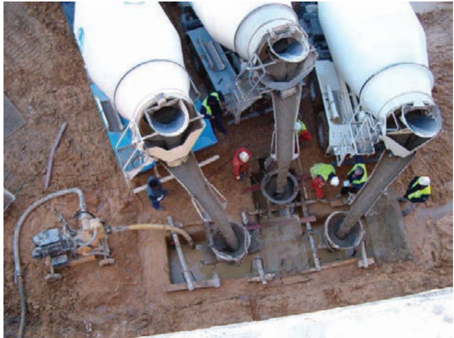
Figura 6. Hormigonado de pantallas con tubo tremi y tres camiones hormigonera. Figure 6. Pouring concrete for the diaphragm walls with tremies and three concrete mixers.
