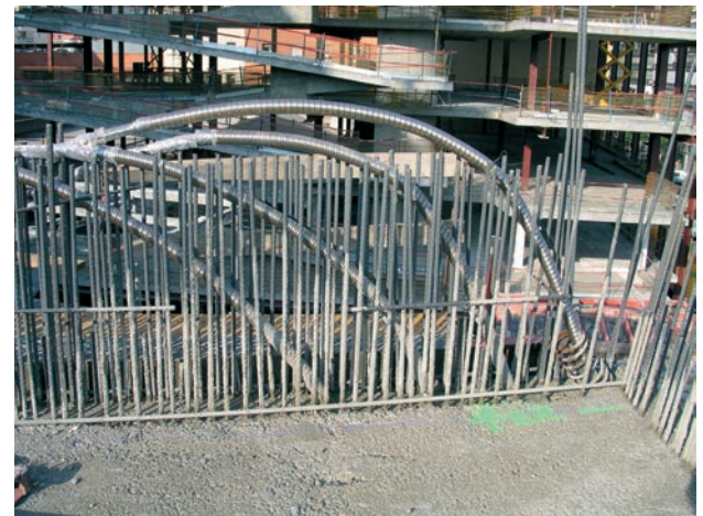
Figura 10. Pretensado de pantallas laterales del Teatro Principal Figure 10. Main Theatre lateral walls prestressing.
