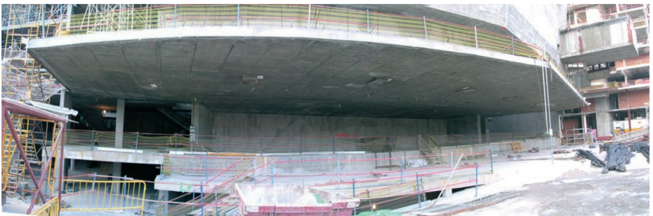
Figura 11. Vista inferior de la gran losa volada del Teatro Principal. Figure 11. Main Theatre cantilever access slab lower view.
