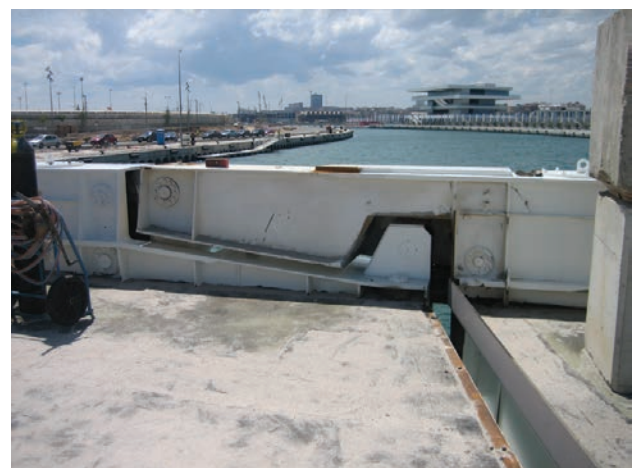
Figura 8. Enclavamiento central. Figure 8. Central interlocking.
