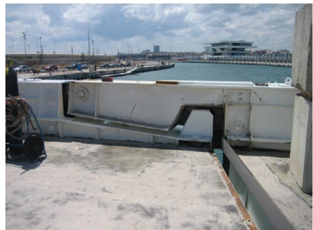
Figura 8. Enclavamiento central. Figure 8. Central interlocking.
