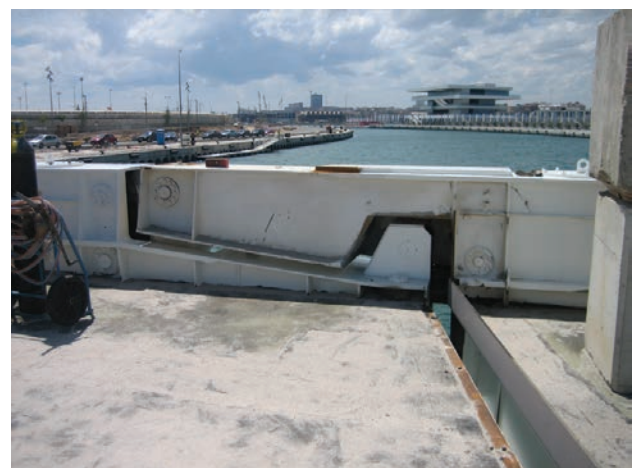
Figura 8. Enclavamiento central. Figure 8. Central interlocking.
