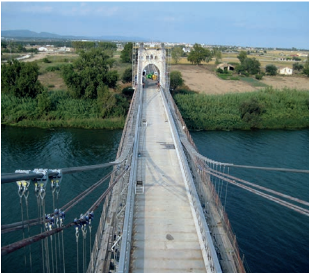
Figura 19. Cables durante la transferencia de cargas del sistema provisional al definitivo. Figure 19. Cables during load transfer from provisional to permanent system.
