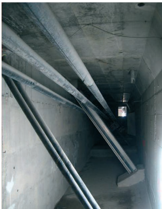
Figura 31. Pretensado longitudinal, diagonales y puntales Figure 31. General view of the external longitudinal prestressing, inclined tensioned bars and inclined supports
