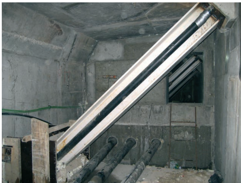
Figura 21. Puntales, diagonales y desviador en centro de vano Figure 21. Inclined internal supports and transverse wall in the centre of the span
