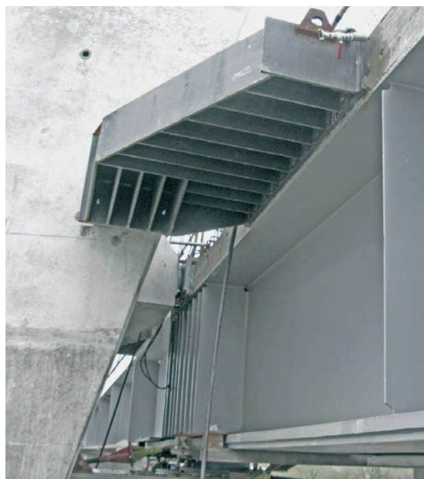
Figura 28. Tope de bloqueo del tablero en la torre Figure 28. Corbel to block the deck movement at the pylon
