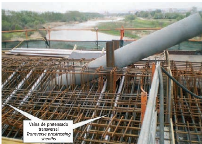
Figura 9. Vainas de pretensado transversal en la salida del tirante Figure 9. Transverse prestressing sheaths around the base of the stay
