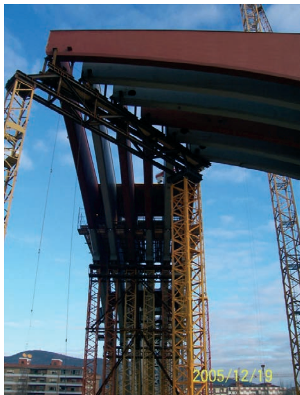
Figura 44. Torres de apeo con celosía superior en las intersecciones Sur-Este y Sur-Oeste Figure 44. Auxiliary supports with upper truss in the South-East and South-West intersections
