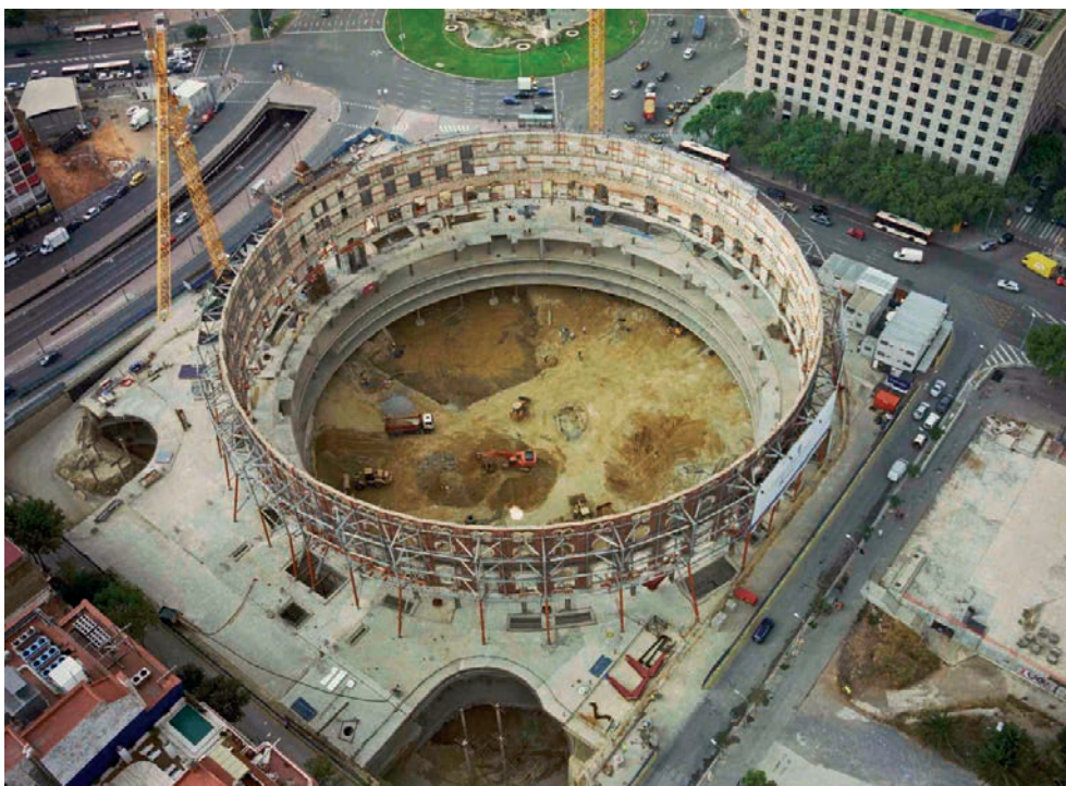
Figura 30. Vista general en la fase de máxima excavación Figure 30. General view during the maximum-excavation stage
