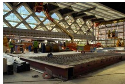
Figure 20. Construction of the steel grid prior to casting the concrete for the composite slab.
