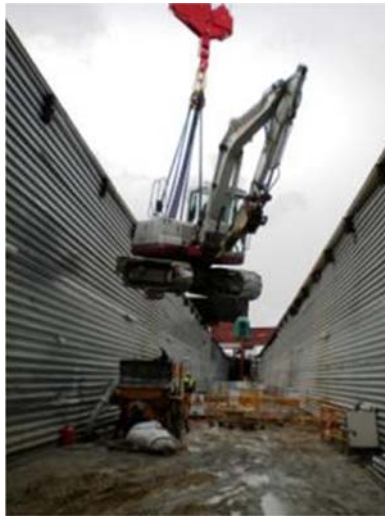
Figure 45. Platform access for machinery.
