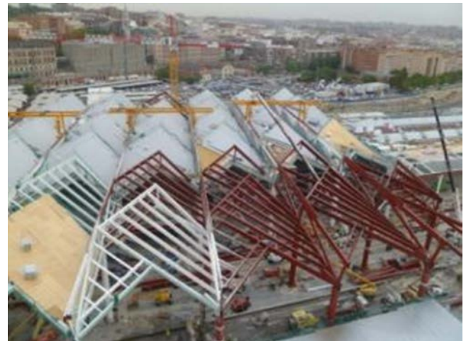
Figure 51. Bridge cranes over the high-rise canopies.
