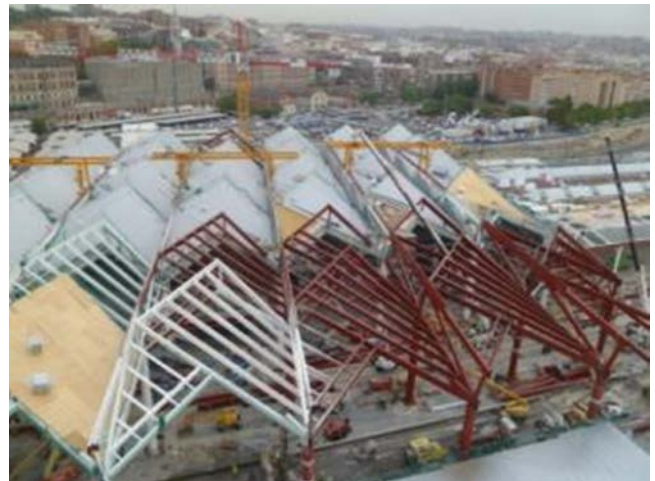
Figure 51. Bridge cranes over the high-rise canopies.
