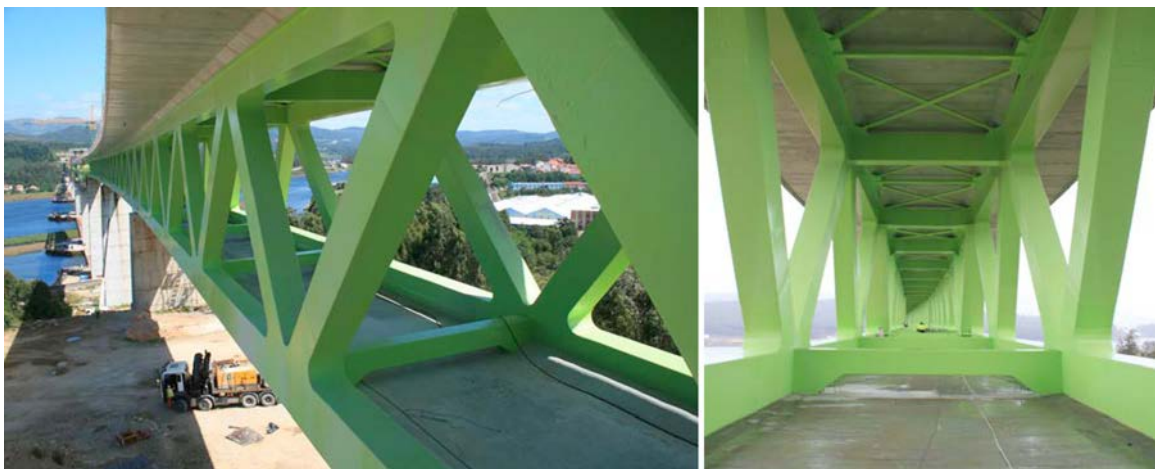
Figure 4. Side view and interior of the truss viewed from the bottom concrete slab.
