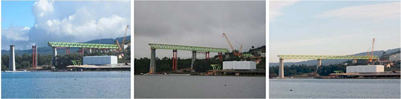
Figure 24. Second stage, 240-m section launched between P3 and P4, and hoisting segments in stage 3.
