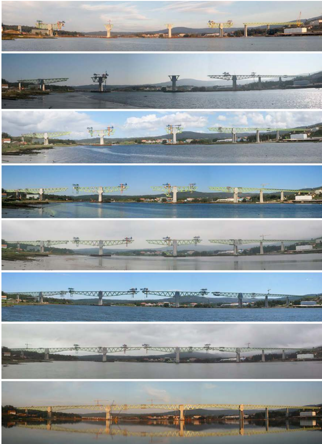
Figure 39. Balanced cantilevering from P5 (right) and P8 (left) and subsequently from P6 and P7.
