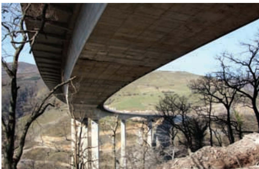
Figura 14. Vista inferior del tablero desde el estribo 2. Figure 14. Underneath view of the deck from abutment 2.
