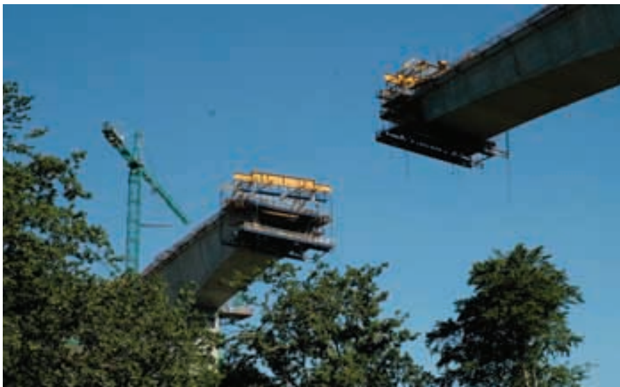
Figura 30. Detalle de carros acercándose en pilas 2 y 3. Figure 30. Detail of travellers approaching each other at piers 2 and 3.
