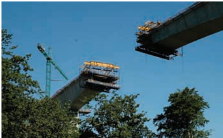
Figura 30. Detalle de carros acercándose en pilas 2 y 3. Figure 30. Detail of travellers approaching each other at piers 2 and 3.
