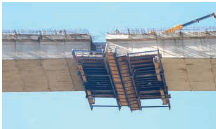
Figura 31. Vista inferior de encofrado de dovela de cierre Figure 31. Underneath view of the connection segment's formwork.
