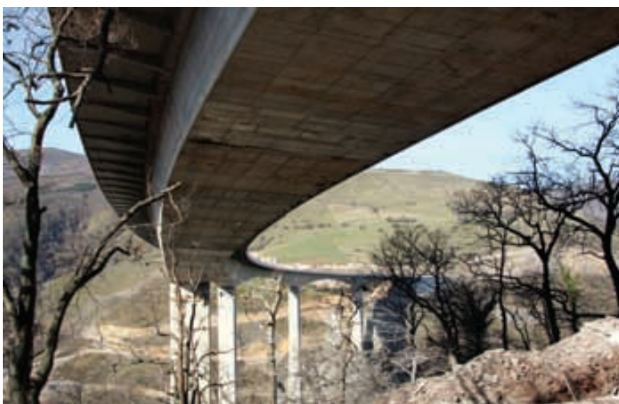
Figura 14. Vista inferior del tablero desde el estribo 2. Figure 14. Underneath view of the deck from abutment 2.
