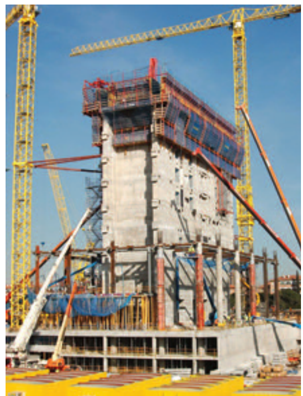
Figura 29. Vista general del arranque de la torre. Figure 29. Lower tower, at springing line.
