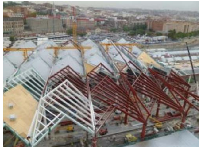
Figure 51. Bridge cranes over the high-rise canopies.
