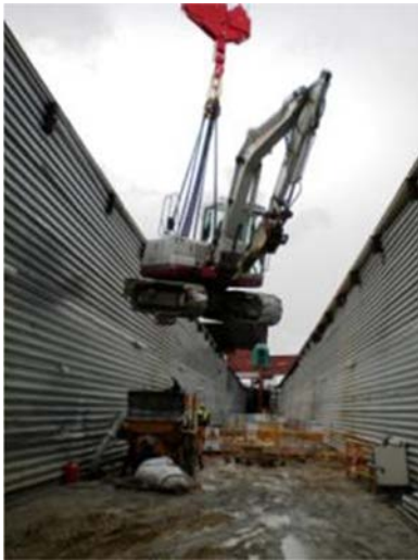
Figure 45. Platform access for machinery.
