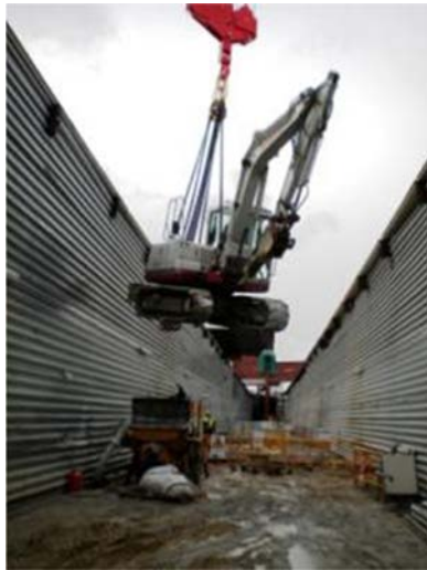
Figure 45. Platform access for machinery.
