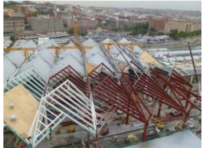
Figure 51. Bridge cranes over the high-rise canopies.
