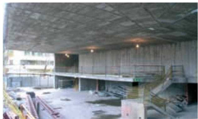
Figura 18. Losa de entrada del Teatro Configurable. Figure 18. Access slab in the Configurable Theatre.
