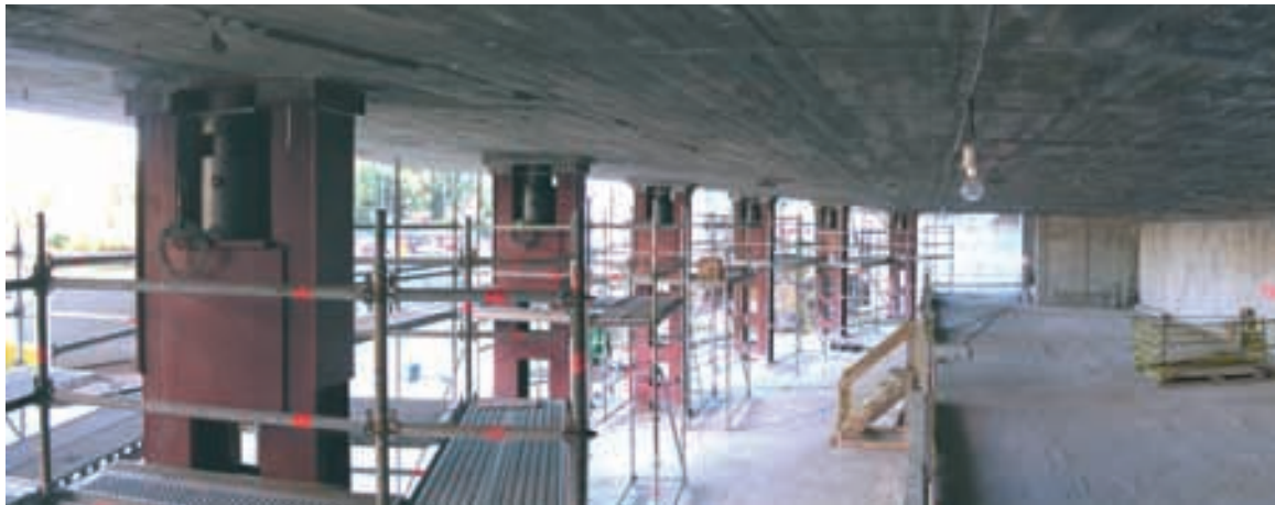
Figura 38. Apeos del Teatro principal con los gatos de desapeo colocados. Figure 38. Hydraulic jacks on the temporary supports of the Main Theatre.
