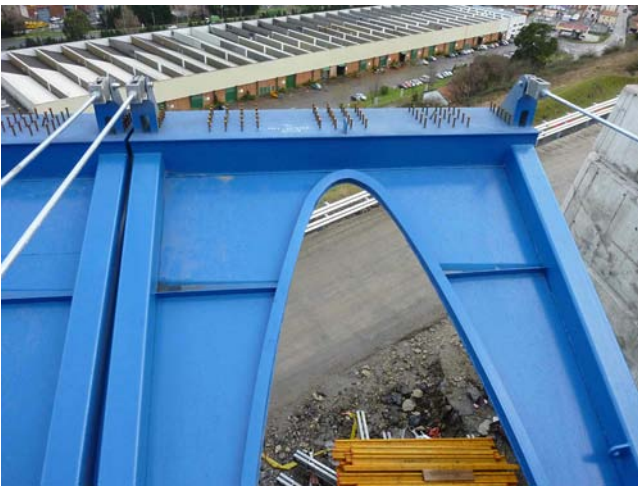
Figures 10 and 11. Main viaduct. Side and front view of the braced box girders.
