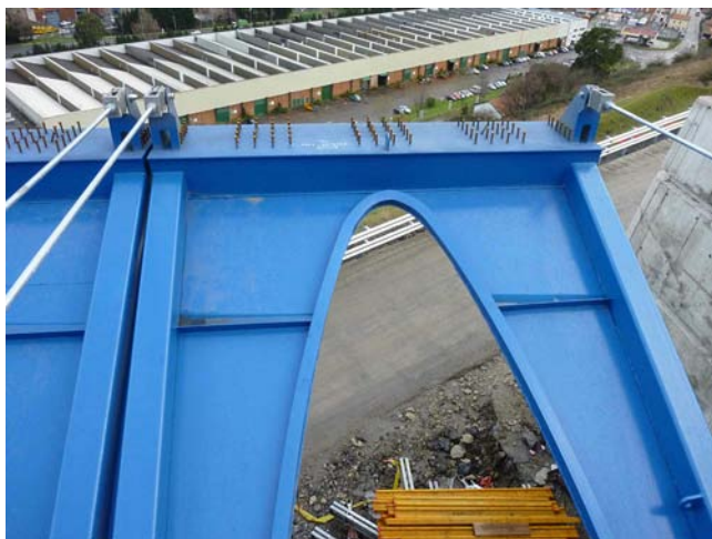
Figures 10 and 11. Main viaduct. Side and front view of the braced box girders.
