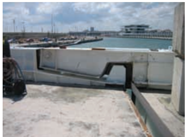
Figura 8. Enclavamiento central. Figure 8. Central interlocking.
