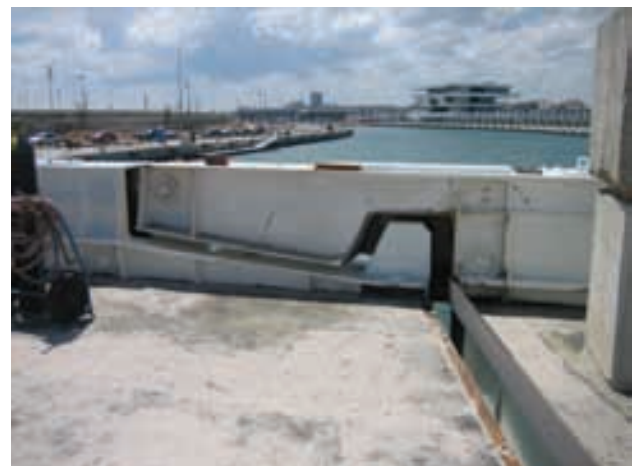
Figura 8. Enclavamiento central. Figure 8. Central interlocking.
