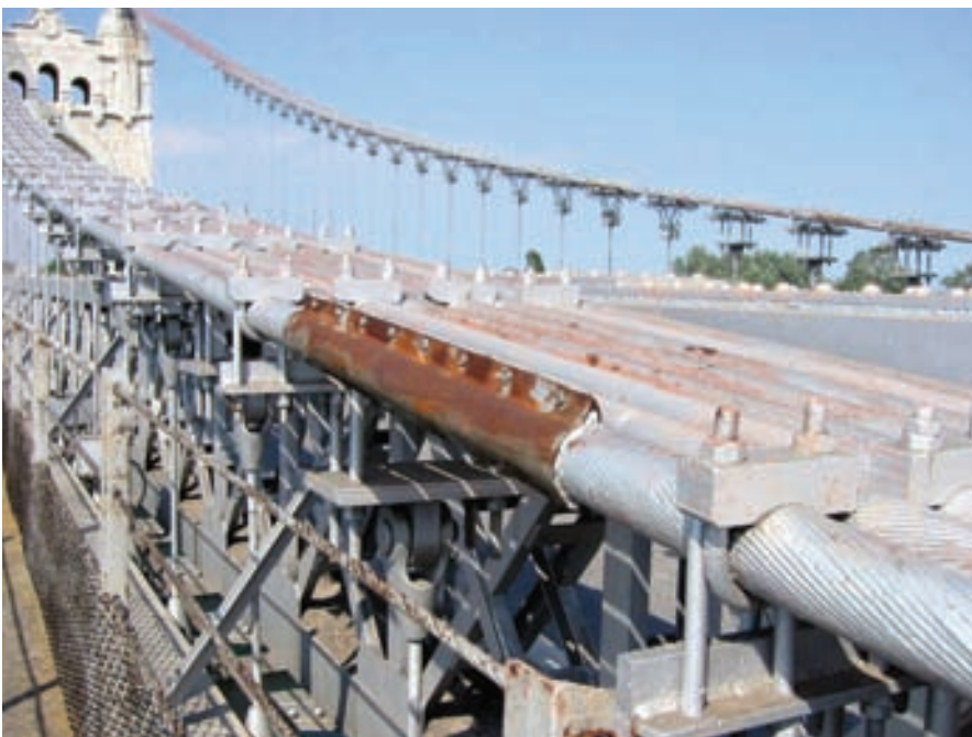
Figura 17. Cables reparados en 1972. Figure 17. Cables repaired in 1972.
