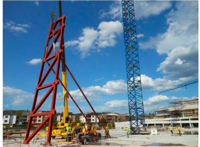
Figure 24. Hoisting the first truss panel: note the provisional props used to stabilise the structure during erection.
