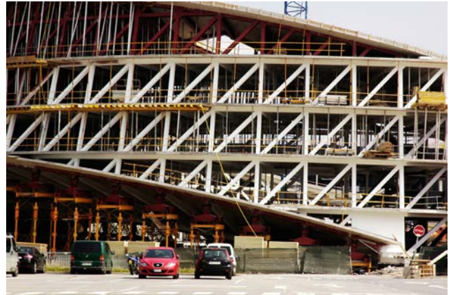
Figure 8. Side view of the outer truss during construction of the structural roof slab: note that the diagonals remain straight at the junction with bottom and roof slabs.
