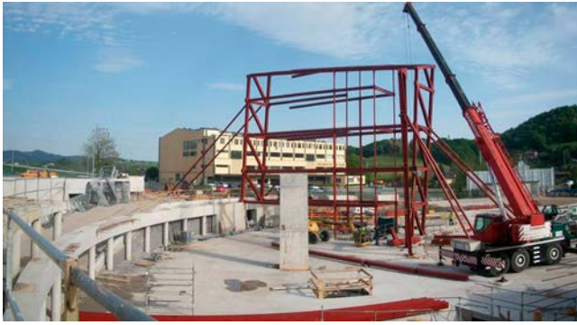
Figure 23. First structural sector, including two opposite truss panels, beams, and intermediate columns, as it was hoisted into position.
