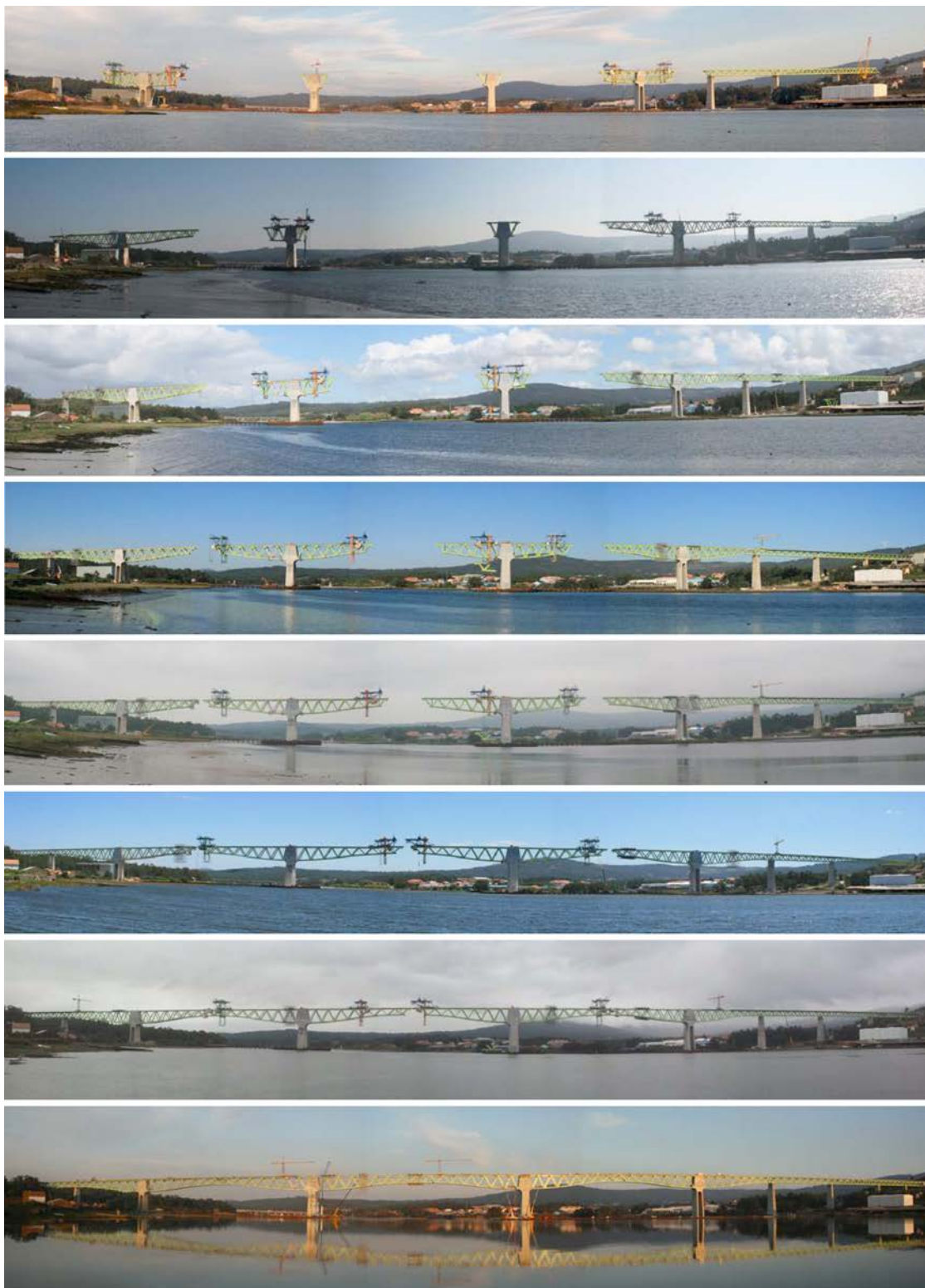
Figure 39. Balanced cantilevering from P5 (right) and P8 (left) and subsequently from P6 and P7.
