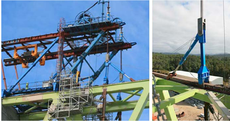
Figure 35. Hoisting a segment with a stationary derrick crane and detail of transverse hoisting beam.
