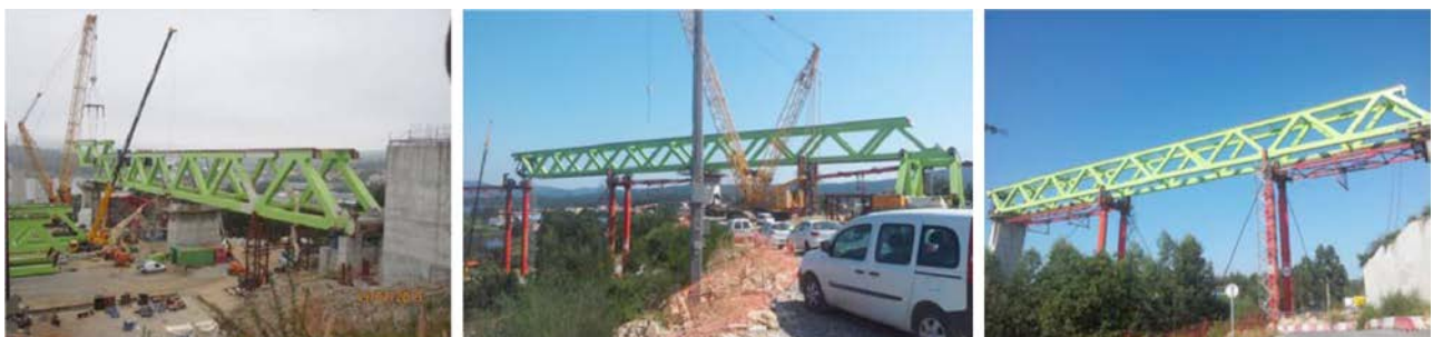
Figure 23. Segment hoisting, first launch and section after launching from P2 to P3.
