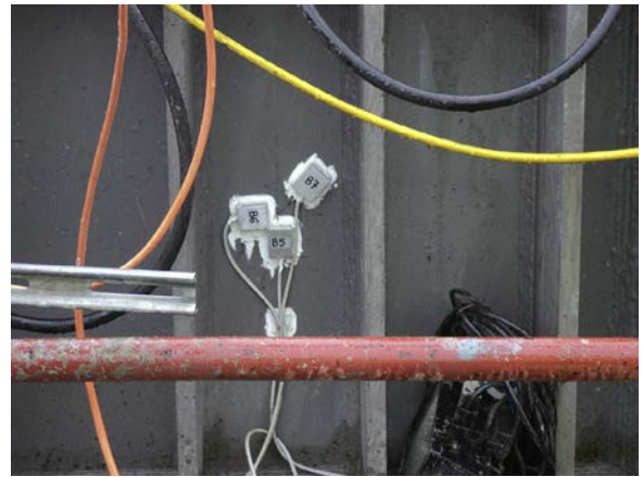
Figure 34. Detail of strain gauges installed on hanger beam webs.
