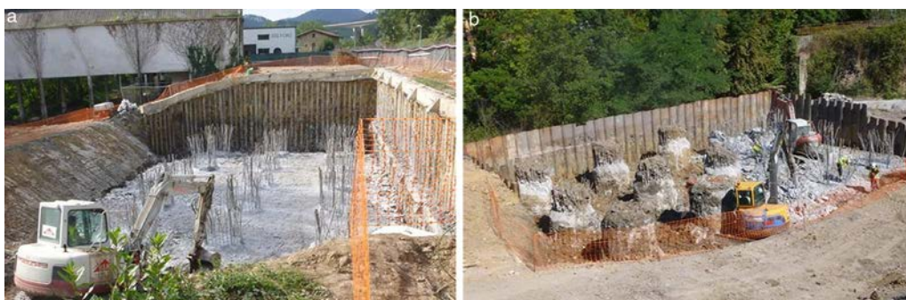
Figure 16. a) Micropile retaining walls for P-7 foundations; b) sheet retaining wall for P-8 pile foundations.
