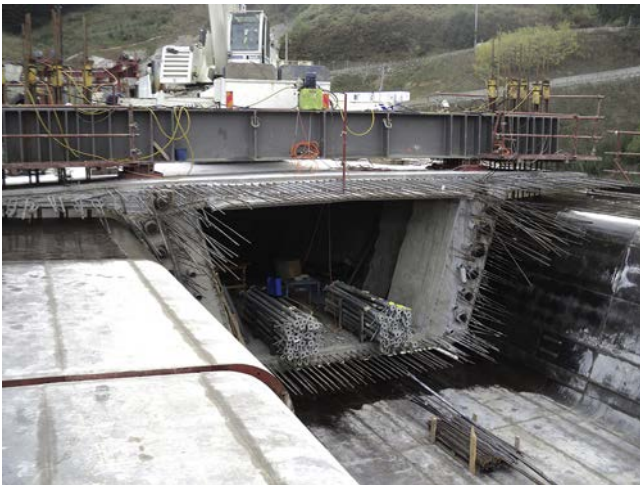
Figure 26. Cantilever front with anchorages for negative reinforcement tendons and parabolic continuity tendons and the system for hanging the MSS from the end of the cantilever.
