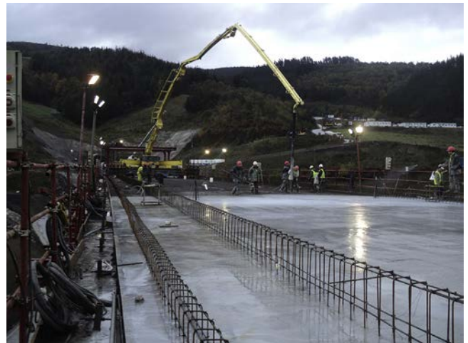
Figure 24. Casting the top slab with concrete pumped from the forward end of the preceding phase.
