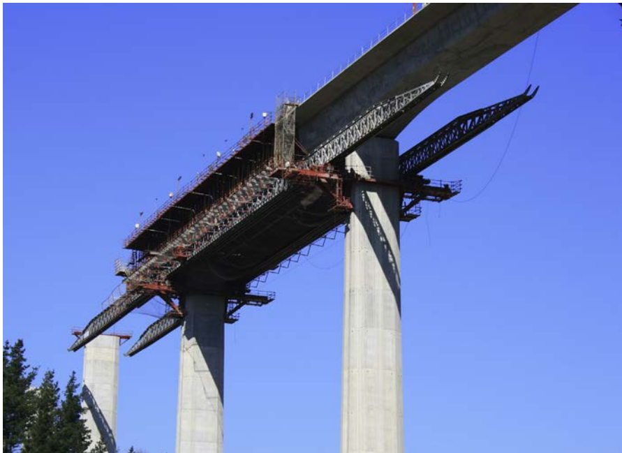
Figure 32. MSS support rings at top of pier.
