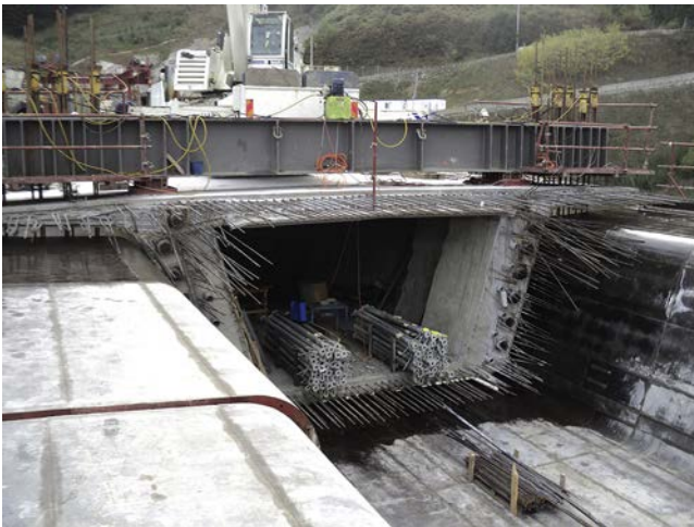
Figure 26. Cantilever front with anchorages for negative reinforcement tendons and parabolic continuity tendons and the system for hanging the MSS from the end of the cantilever.
