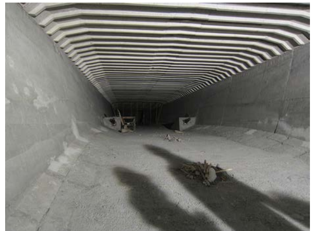
Figure 27. Inside of deck with anchorages for positive reinforcement prestressing in background.
