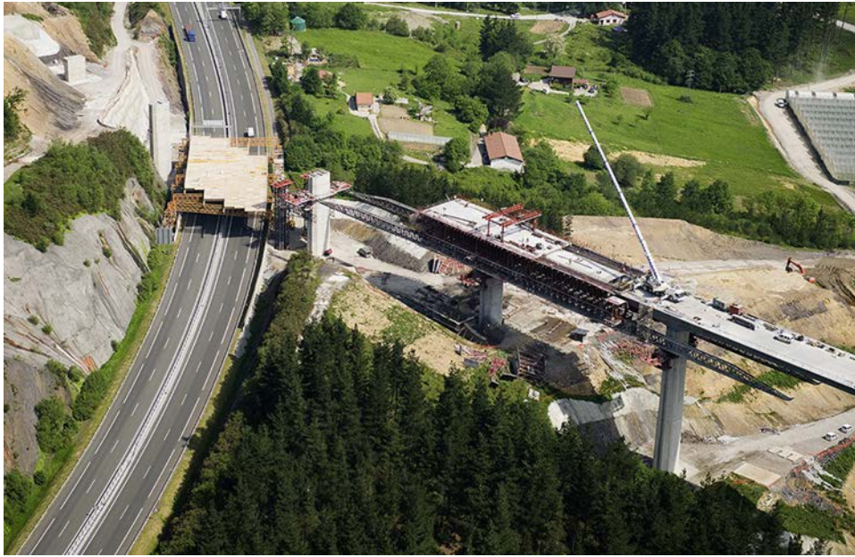
Figure 25. Overview of area of negative reinforcement completely cast in concrete and laying of precast slabs in the positive reinforcement section, for subsequent assembly and concrete casting of the top slab rebar.
