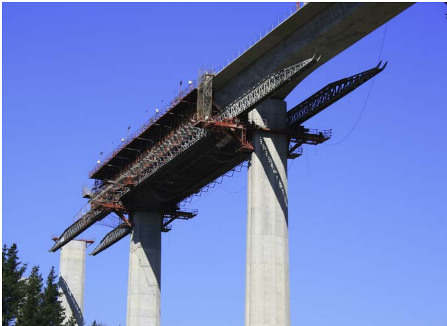
Figure 32. MSS support rings at top of pier.
