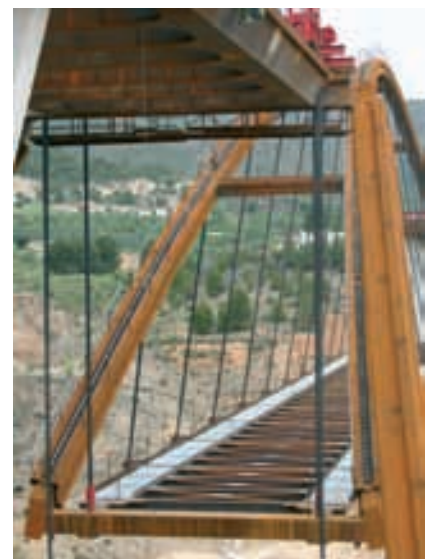
Figure 21. Riostra de bowstring Figure 21. Bowstring brace
