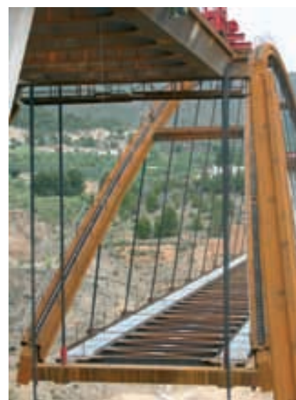
Figure 21. Riostra de bowstring Figure 21. Bowstring brace
