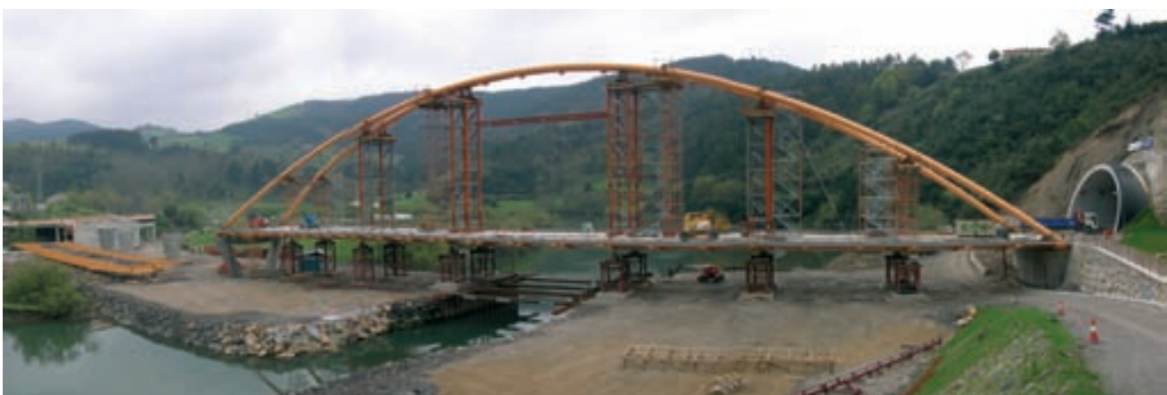
Figura 28. Vista del arco y tablero apeados Figura 28. View of the arch and deck while shored
