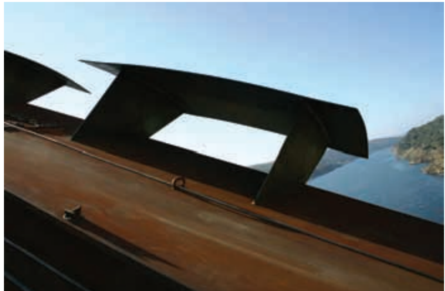
Figura 58. Deflector. Detalle. Figure 58. Guide vane. Detail.
