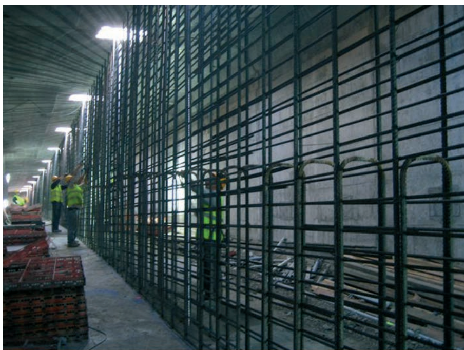
Figura 30. Ferrallado anterior al hormigonado del alma central Figure 30. Installing the reinforcement, before the central web was poured.
