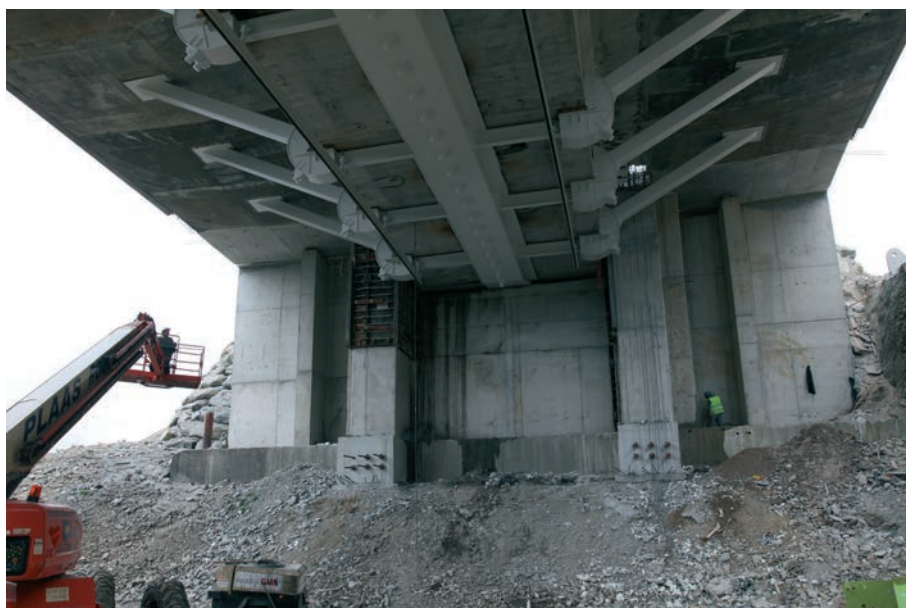
Figura 28. Vista general del estribo una vez reforzado Figure 28. General view of the abutment once it was reinforced
