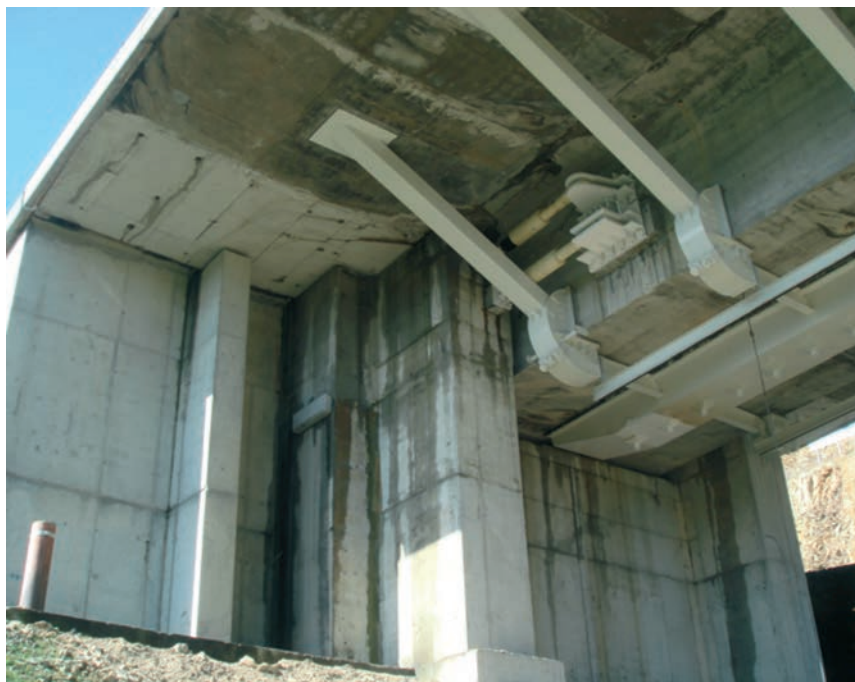
Figura 11. Vista general del estribo y dispositivos transmisores de carga Figure 11. General view of the abutments and of the shock transmission devices
