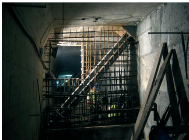
Figura 34. Ferrallado de desviadores Figure 34. Reinforcing of the transvers walls of the deck
