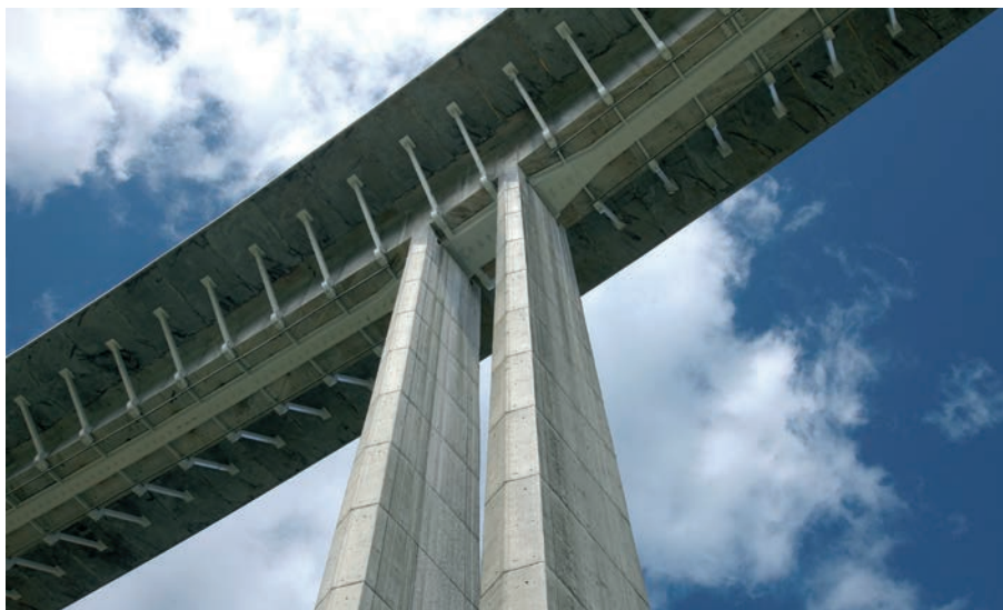
Figura 7. Solución II, refuerzo de cajón existente. Vista inferior del tablero ampliado Figure 7. Solution II, reinforcing of the existing deck. Lower view of the widened deck
