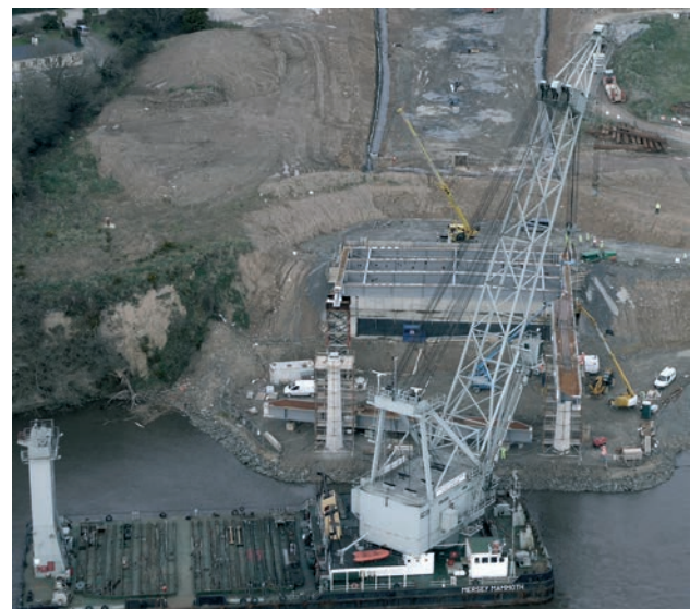
Figura 39. Colocación del tramo de espera mediante grúa flotante Figure 39. Installation of the end span by a floating crane
