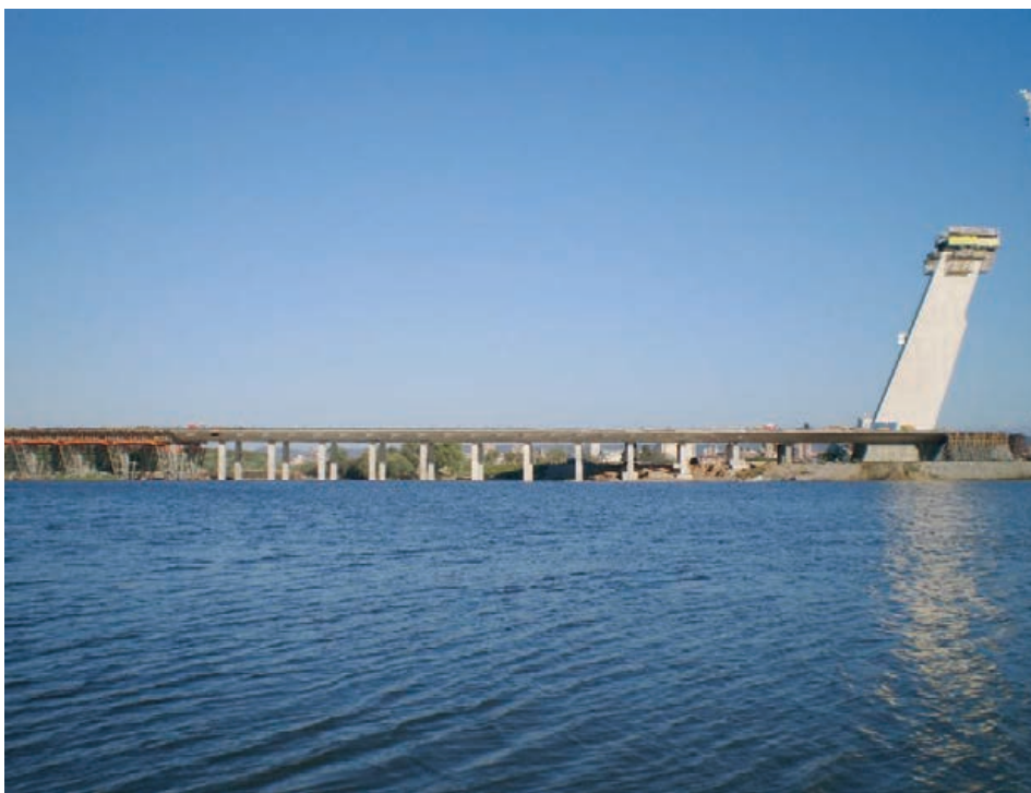
Figura 35. Tablero apoyado sobre pilas provisionales y pilono antes de colocar los cables Figure 35. Deck resting on provisional piers and pylon before cables were strung
