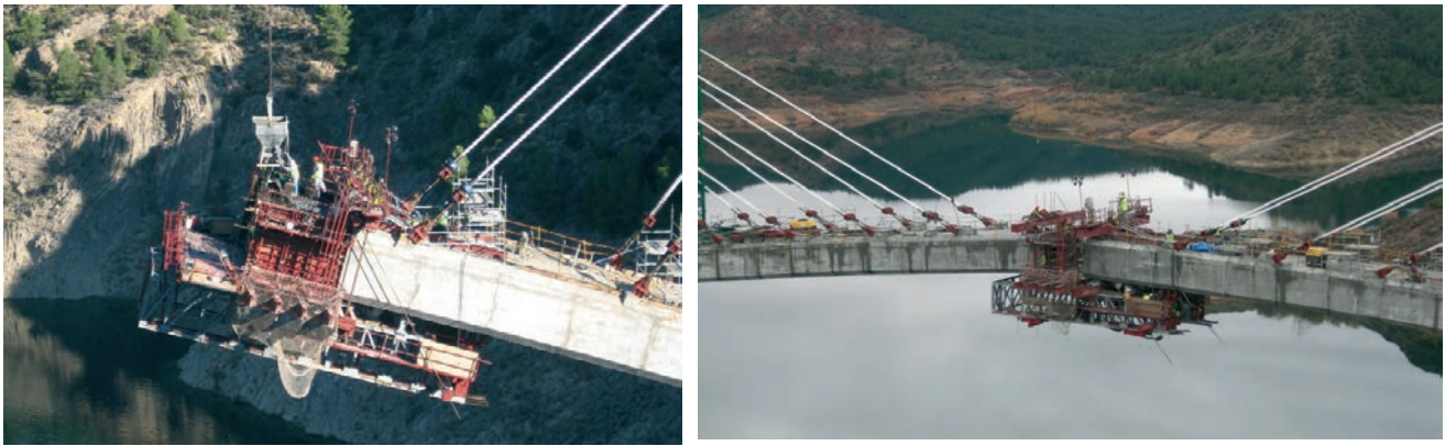
Figura 20. Detalles del carro de avance y del cierre en clave Figure 20. Details of the form traveller and the connection at the key
