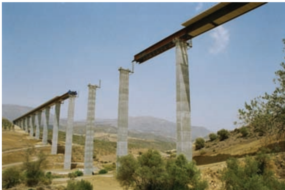
Fig. 31. Vista de pilas durante el empuje. Fig. 31. View of piers during launching.
