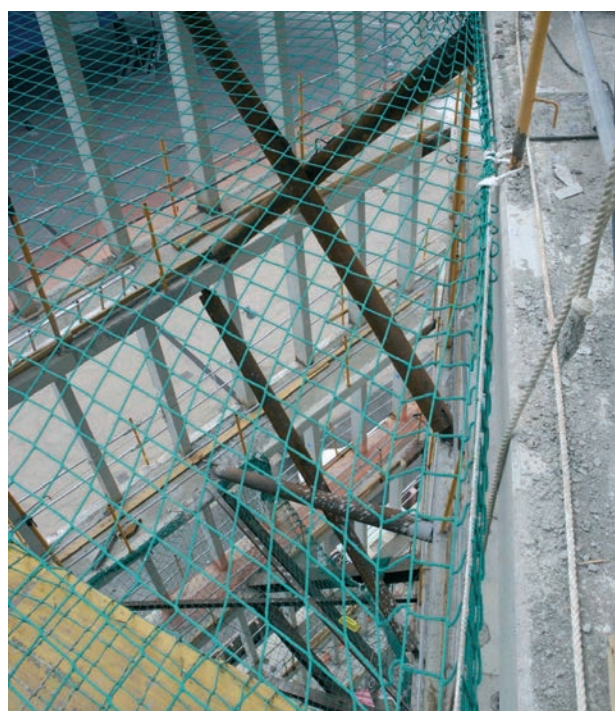
Figura 30. Arriostamiento provisional capa interior fachada en patio Figure 30. Provisional shoring of the inner layer of the facade surrounding the lower patio
