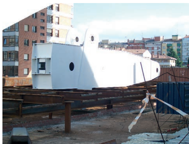
Figura 30. Palanca guiadora antes de ser instalada en el foso Figure 30. Lever arm before its installation in the housing of the cylinders
