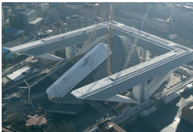
Figura 4. Vista aérea durante las obras del Conjunto de Edificaciones Buenavista Figure 4. Aerial view of the Buenavista Building Complex during the construction works
