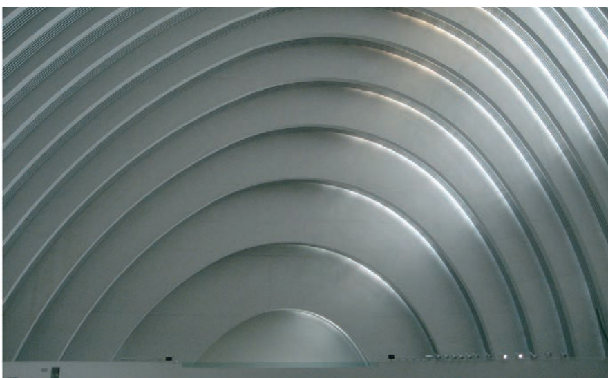
Figura 7. Bóveda superior de la sala mayor del Palacio de Exposiciones y Congresos Figure 7. Top vault of the main auditorium of the Congress and Exhibition Center
