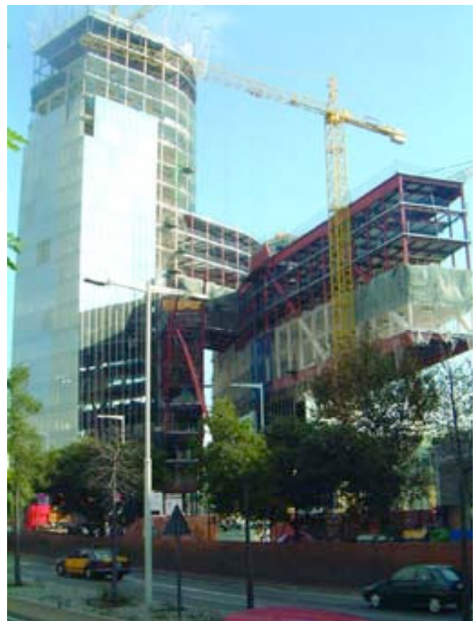
Figura 30. Vista general en fase de terminaciones. Figure 30. General view of finishing work.
