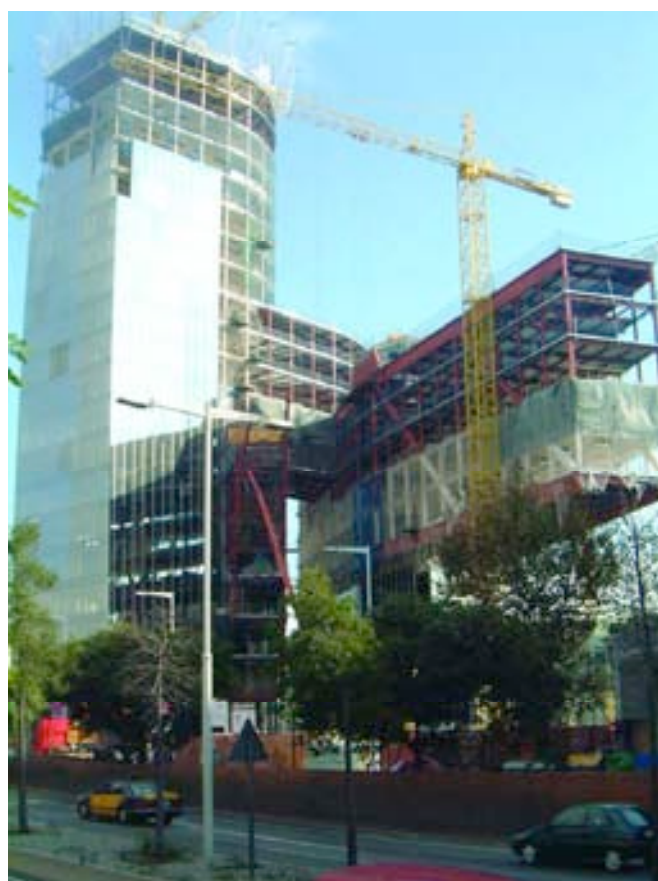
Figura 30. Vista general en fase de terminaciones. Figure 30. General view of finishing work.
