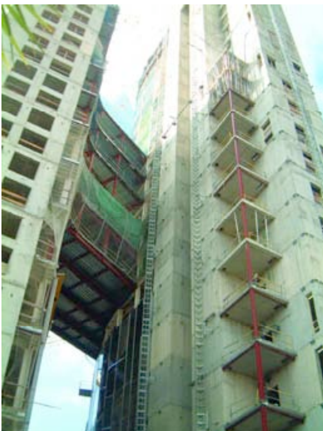
Figura 29. Vista dorsal de la Torre y el Puente. Figure 29. Rear view of the Tower and Bridge buildings.
