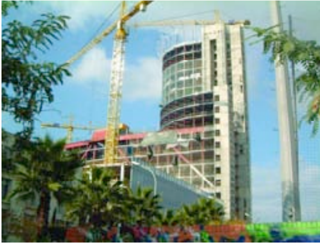
Figura 31. Vista dorsal en fase de cerramiento. Figure 31. Rear view during construction of facings.
