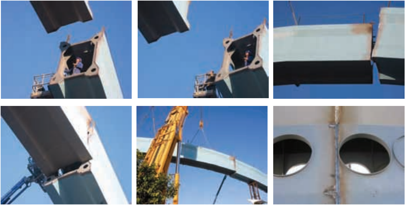
Figuras 37. Uniones a tope de los cajones. Figure 37. Butt joints of the caissons.
