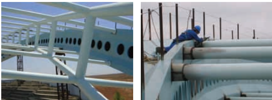
Figura 39. Uniones terminadas de tubos y cajón con teja y contra-teja. Figure 39. Finished joints of the tubes and caisson with dowels and counterdowels.
