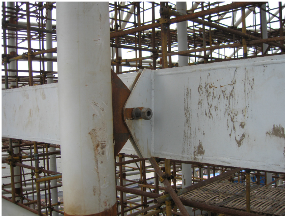
Figura 17. Unión bulonada en construcción, conectando viga de borde con tubo de fachada mediante orejetas Figure 17. Pin-bolt connection under construction, connecting the floor edge beam to the facade tube through ear-plates
