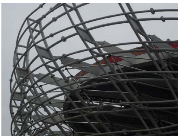
Figura 20. Detalle de la cubierta de la Sala Expositiva 2. Las vigas triangulares se unen por medio de bulones a la fachada, rigidizada por paneles en esa zona Figure 20. Detail of the roof of Exhibition Room 2, where the triangular beams are connected through pin-bolts to the facade, reinforced in this area with plates
