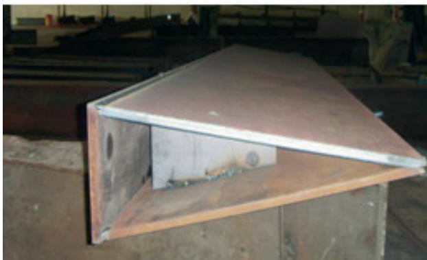
Figura 19. Viga triangular en construcción en taller (tumbada) Figure 19. Triangular beam under manufacture at the workshop (turned)
