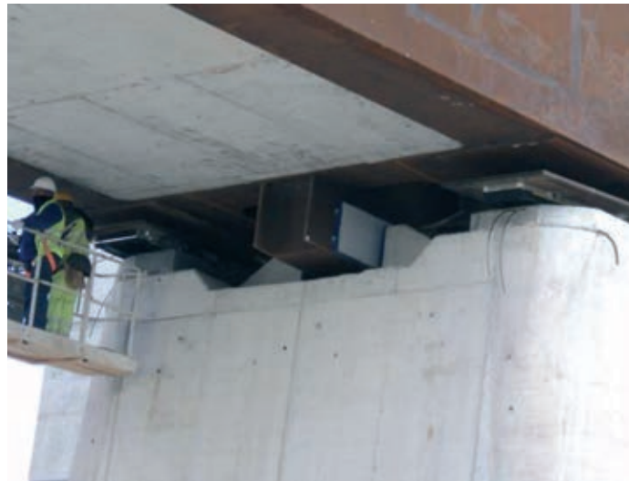
Figura 29. Vista inferior del tope sísmico y aparatos de apoyo en estribo Figure 29. Lower view of the seismic shearkey and bearings at abutments
