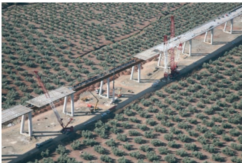
Figura 27. Vista general del montaje de la losa Figure 27. General view during slab assembling
